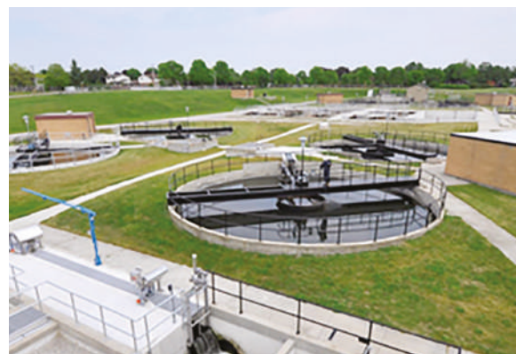
Goderich Water & Wastewater System Ontario
